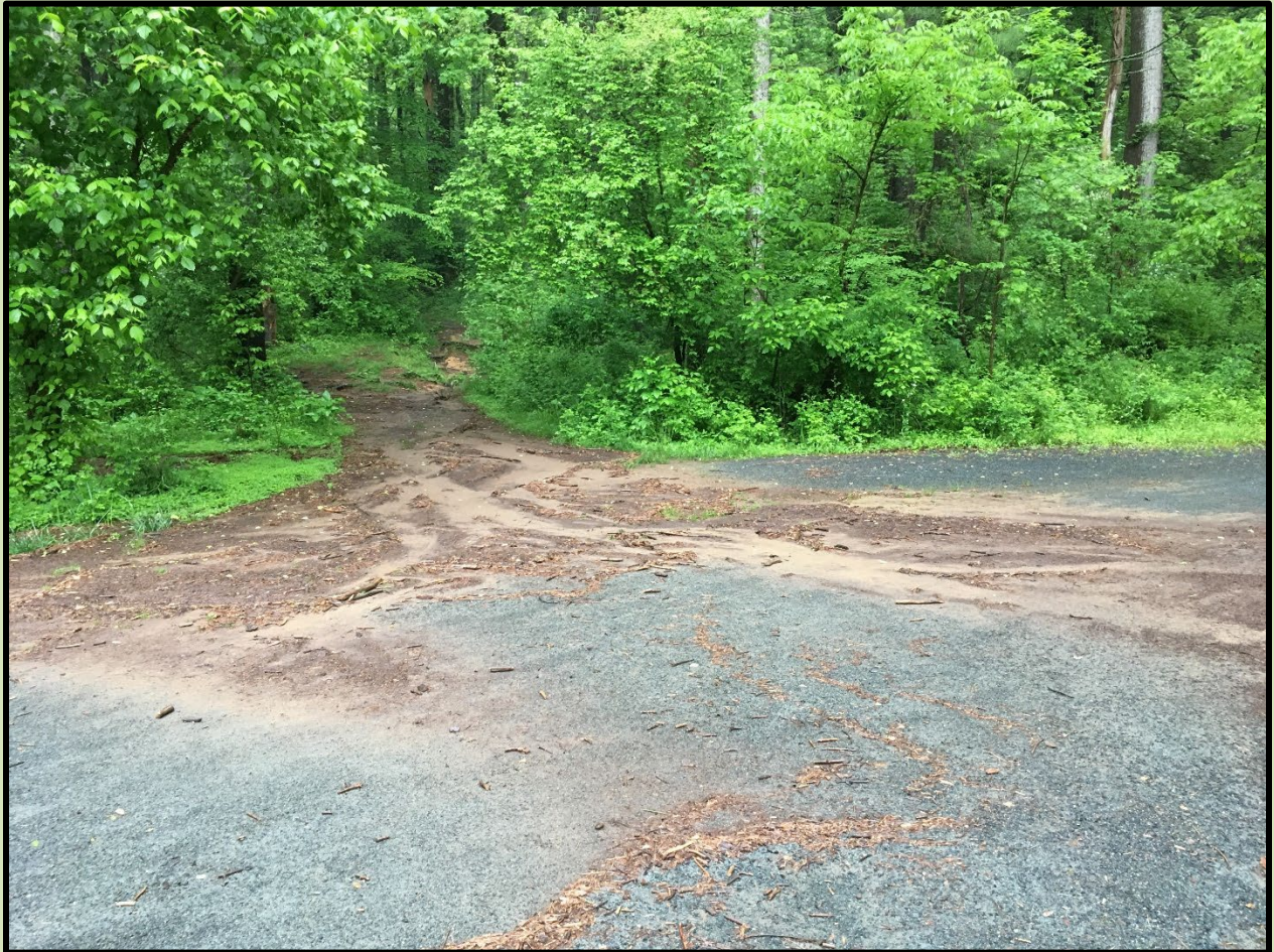
Erosion at the Intersection of Rocky Run and Brandywine Trails
