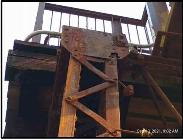
Figure 7: Pier 1, west vertical post contains open crack at the top gusset plate. Diagonal lattice bracing is missing rivets in several locations.
