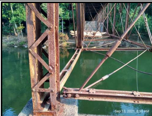
Figure 12: The East and West Trusses are bowing to the east. West Truss shown, West Truss similar.
