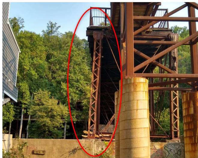
Photo 10: Pier 1 West post shifted towards East
