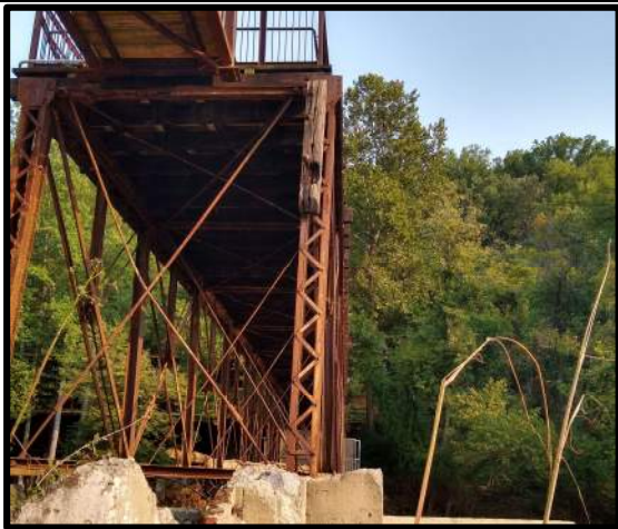
Figure 9: Pier 1 east vertical post is leaning to the east.
