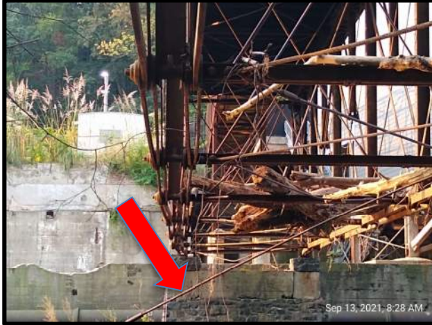
Figure 1: Bottom diagonal tie-rod in fifth bay is broken on one end and hanging down.
