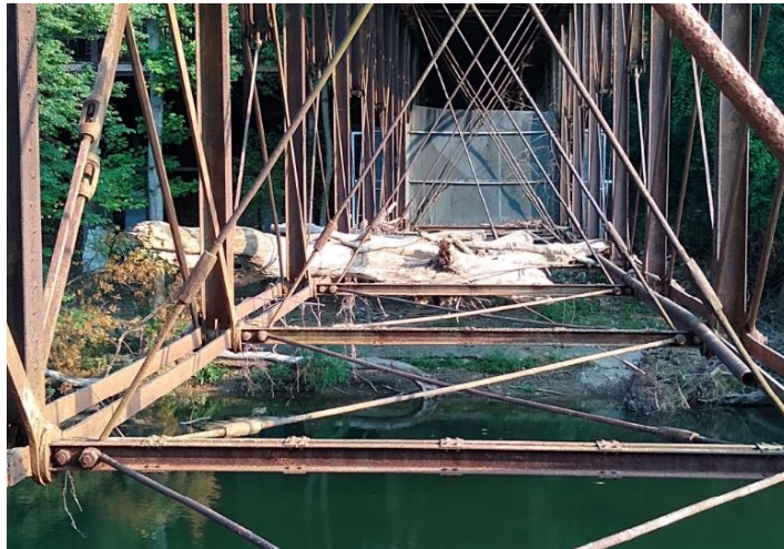
Photo 9: Large tree limbs and debris stuck at bottom chord of the deck trusses with broken tie-rods
