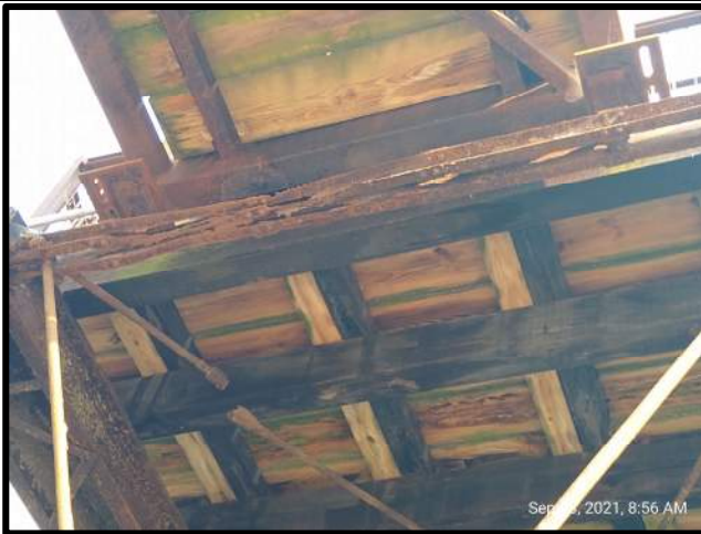
Figure 11: The south end of Main Truss top horizontal member is severely rusted with extreme section loss. This element provides no structural support.
