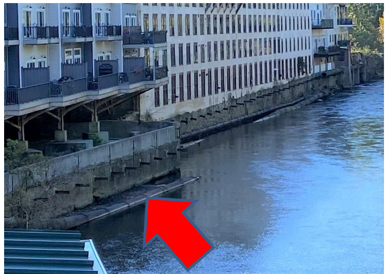
Photos 12 and 13: Water main along the South edge of the creek
