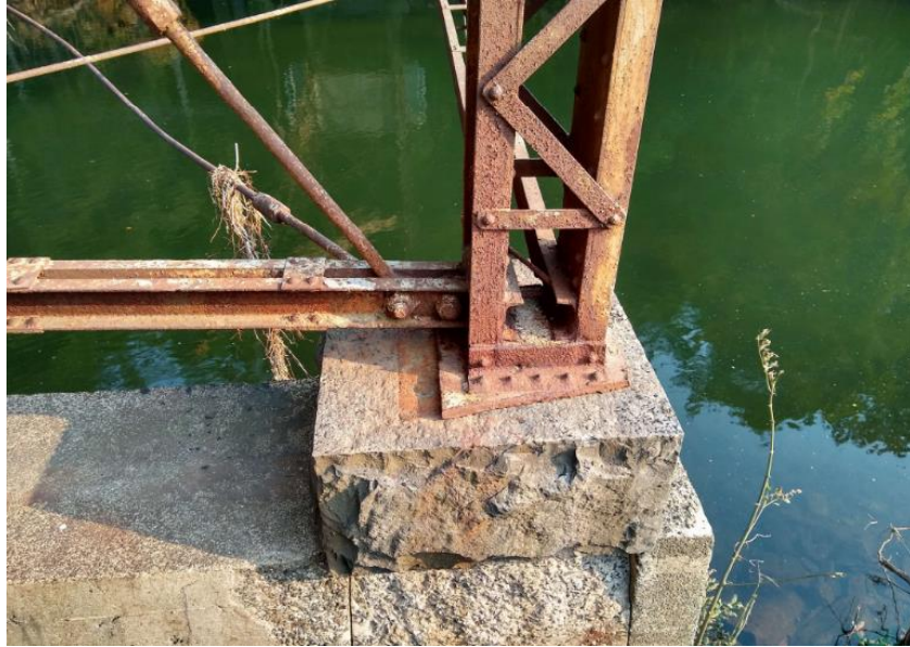
Photo 6: Pier 1 East post sheared off at the anchor bolts and has moved 4.5 inches
