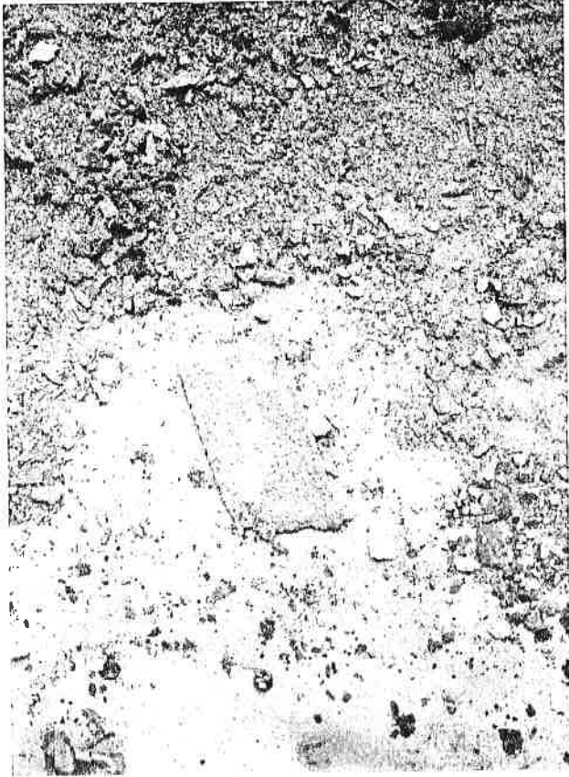
PHOTO #5-Portion of delaminated beam flange that has fallen from structure above.
