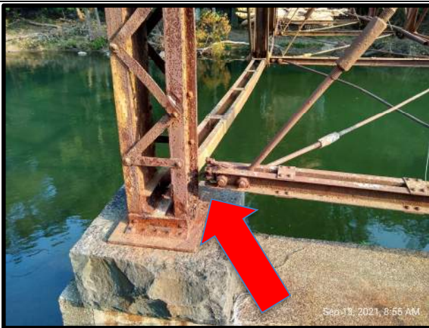
Figure 5: Pier 1, bottom horizontal double channel is cracked and separated from the west post.
