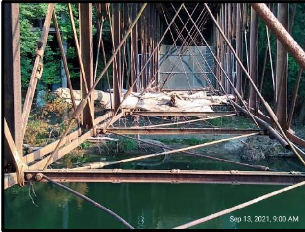
Figure 10: Large tree limbs and debris are hung-up in truss.
