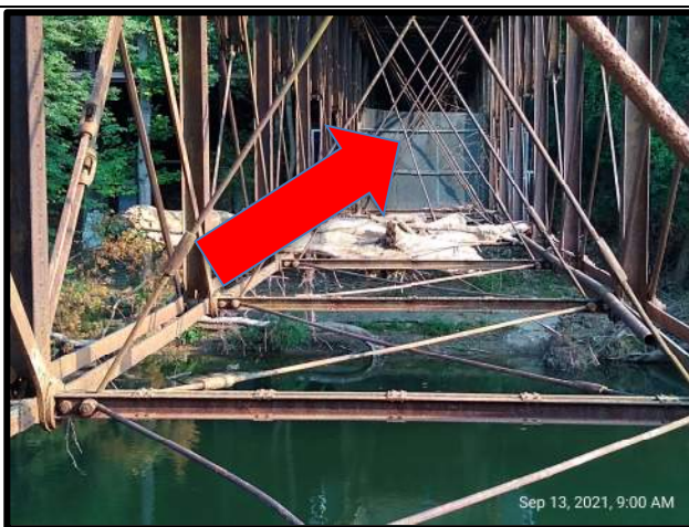
Figure 3: Diagonal tie-rod in 4 th bay connecting top west chord to bottom east chord is broken at the bottom and hanging from the top.
