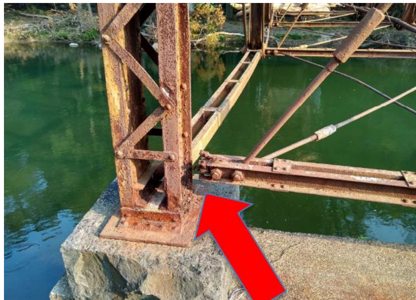
Photo 7: Pier 1 Bottom horizontal separated from west post
