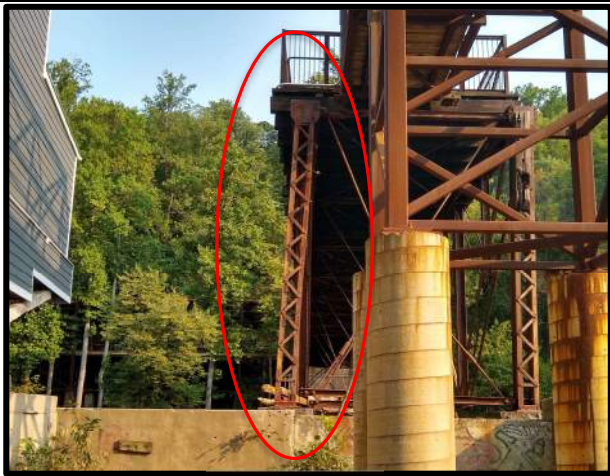
Figure 8: Pier 1 west vertical post is leaning to the east.
