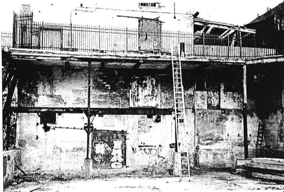
PHOTO #1-Elevation view of bridge approach showing corroded steel frame and existing mill building beyond.
