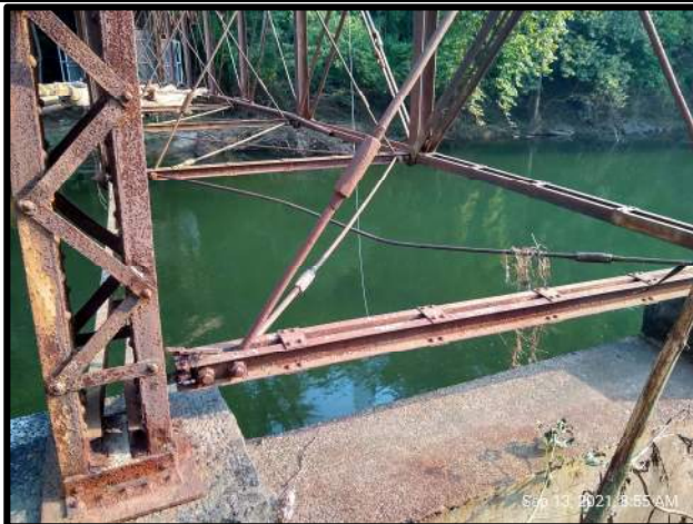
Figure 2: Bottom diagonal tie-rod in first bay is severely bent from compression caused by the west truss shifting to the east.
