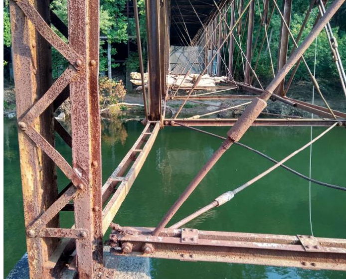
Photo 8: Bowing of the upstream and downstream trusses due to debris damage
